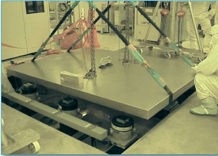
Installation of a TMC Quiet Island® with a high stiffness, highly damped stainless steel platform on STACIS®. (Photo courtesy of Texas Instruments' Kilby Center)
